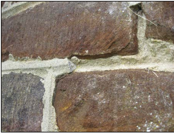
FIG. 24: Heathstone. Blocks of heathstone seen at the parish church. This detail shows failure of poor quality pointing, the raised and smeared appearance of which has greatly disfigured the appearance of the building and may have accelerated decay of the stonework.
