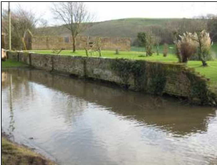
FIG. 17: Garden wall opposite East Creech Farm. The brickwork is in poor condition, being damaged by ivy and leaning in places.
