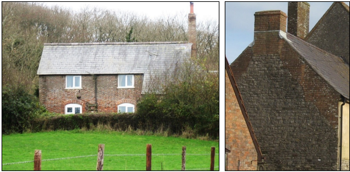
FIG. 5: Increases in height. Both Keeper's Cottage (left) and the west side of East Creech Farm (right) show signs of a historic increase in height. At Keeper's Cottage the band of brickwork at first floor level is a different colour to that below, whilst brick has similarly been added above stone at the farmhouse. Each carries a slate roof though given the age of the buildings the original coverings would have been different. Keeper's Cottage may have originally been a single storey thatched dwelling.
