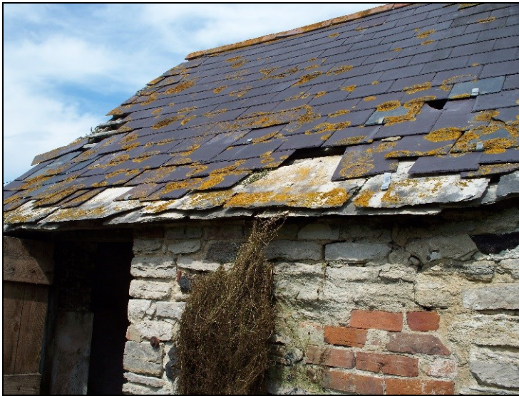
FIG. 11: Welsh slate and stone eaves course. This photo captures roofing materials and details recently lost in the poorly handled conversion of the small agricultural building opposite East Creech Farm. The detail can still be viewed in combination with clay tiles on the farmhouse itself. Note the wall shown here has also been insensitively rebuilt.
