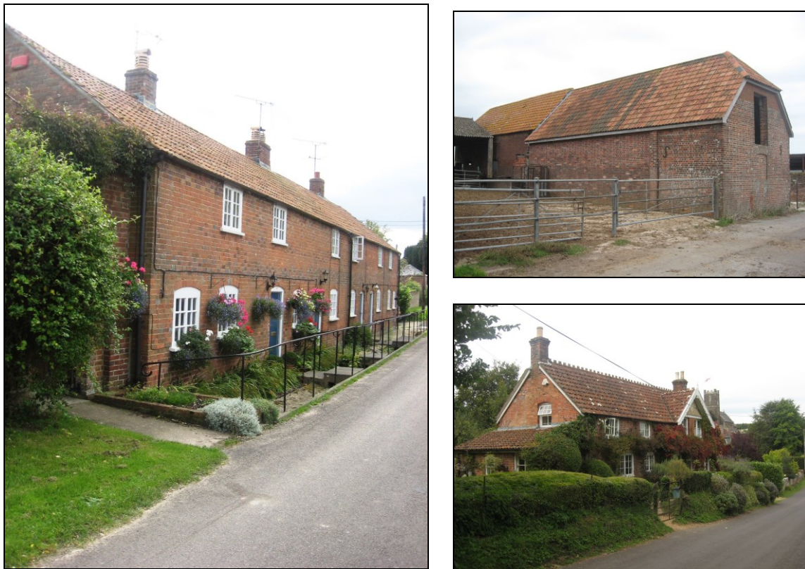
FIG. 31: Double Roman tiles. As seen on the roofs of Nos. 64-67 Higher Street (left), a building at Hill Farm (top right) and the Old Post Office Higher Street (bottom right).
