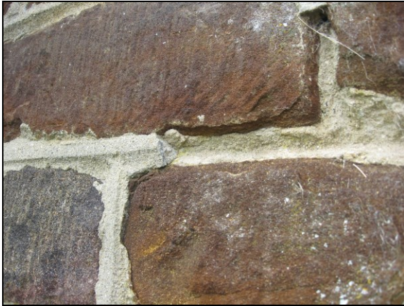
FIG. 23: Heathstone. Blocks of heathstone seen at the parish church. This detail shows failure of poor quality pointing, the raised and smeared appearance of which has greatly disfigured the appearance of the building and may have accelerated decay of the stonework.
