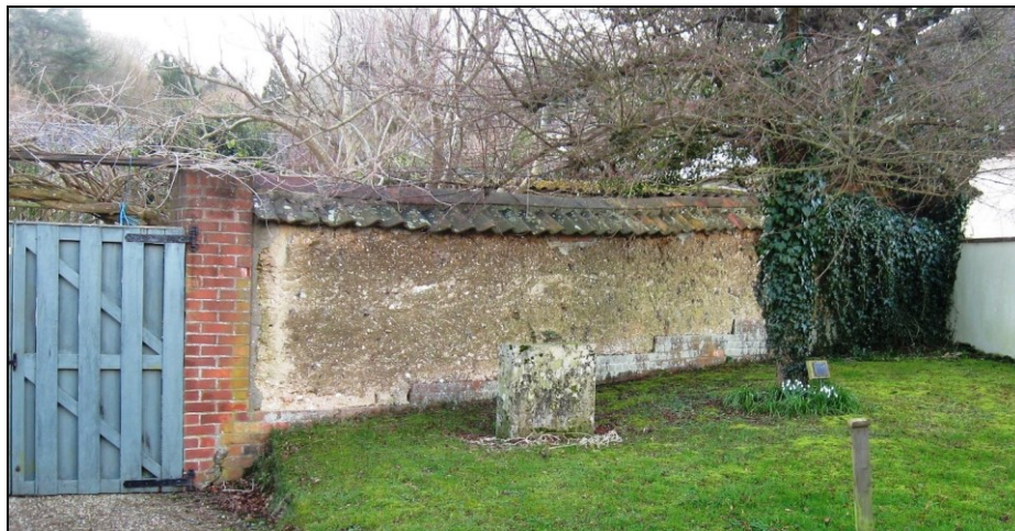
FIG. 20: Section of cob boundary wall, Briantspuddle. The protective coat of render appears to have fallen off or been removed. Note the pantile coping and brick plinth.
