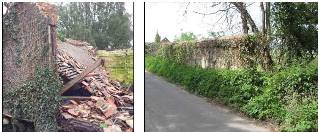
FIG. 37: Derelict buildings and structures. Left: the listed granary at East Farm, Affpuddle. Right: ivy covered remnants of a cob boundary wall, Affpuddle.
