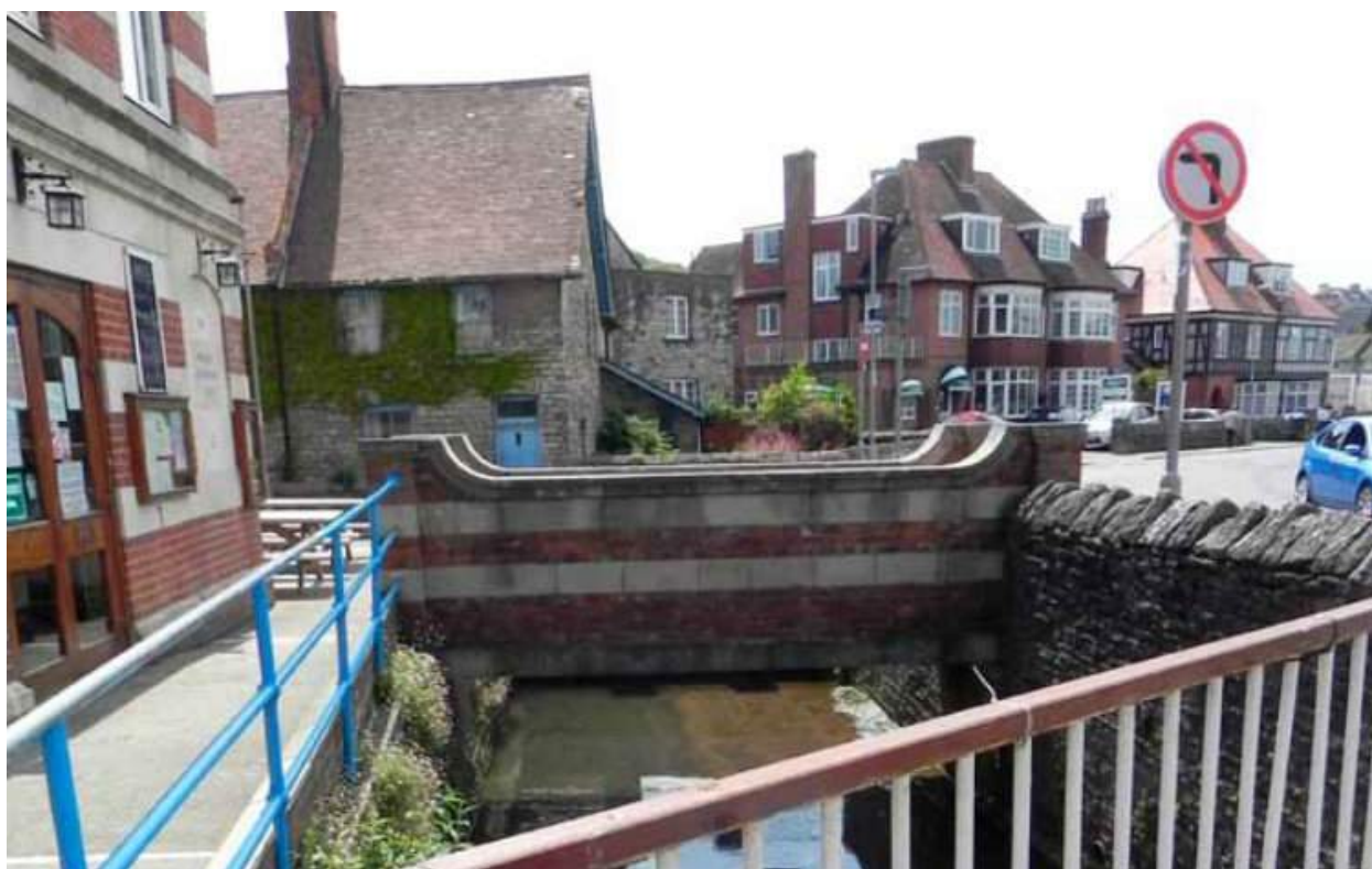
The Swan Brook outside the main Post Office is contained in channel and is culverted under Station Road re-emerging adjacent to the Mowlem
